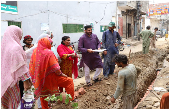
Shakeela, inspecting the work in progress with other members of the community
